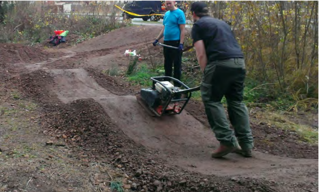
Step 5 – A plate compactor is used to compress the dirt into a a rideable surface. At this point the track is given a test ride to ensure the track maintains a consistent, usable flow.
