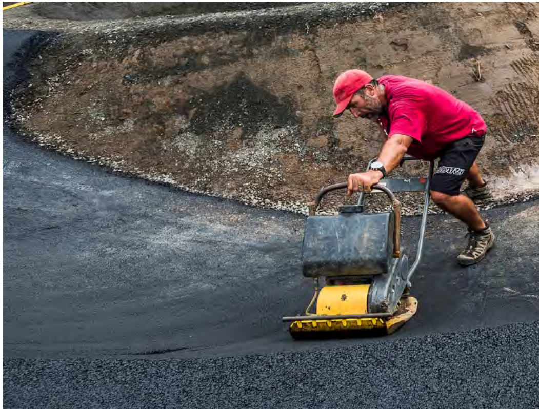
Step 6 – Once the track has been tested and confirmed to ride correctly, the final step is to cover the track with an asphalt surface.
